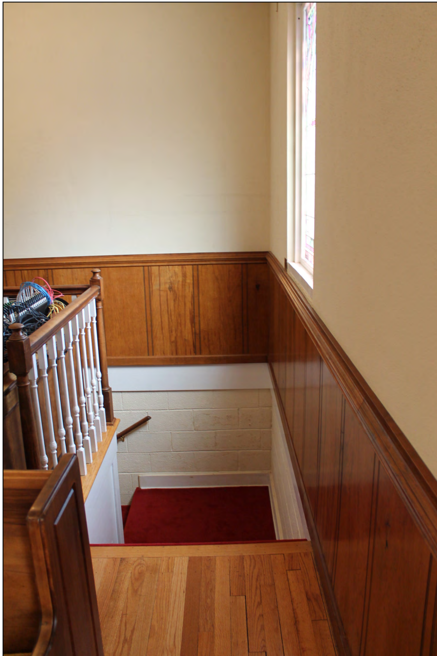
Figure 4.13: Sorrell's Grove Baptist Church (WA8802), stair to basement in north front corner of sanctuary.
